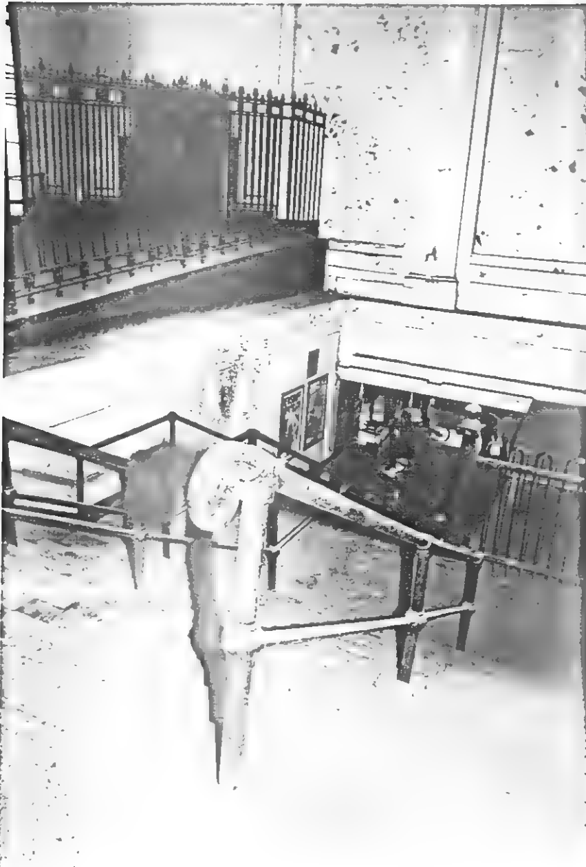
Iron railing separates stairway of corridor leading from ferry concourse to track level and ramp leading to YMCA Building.
